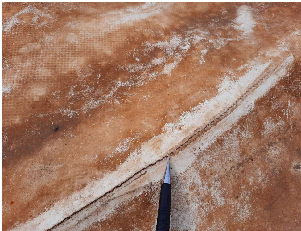
FIGURES 12–13 Surface cracks found in the RPP liner material folds and creases
