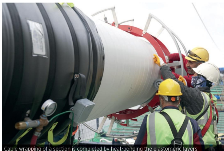
Cable wrapping of a section is completed by heat-bonding the elastomeric layers
