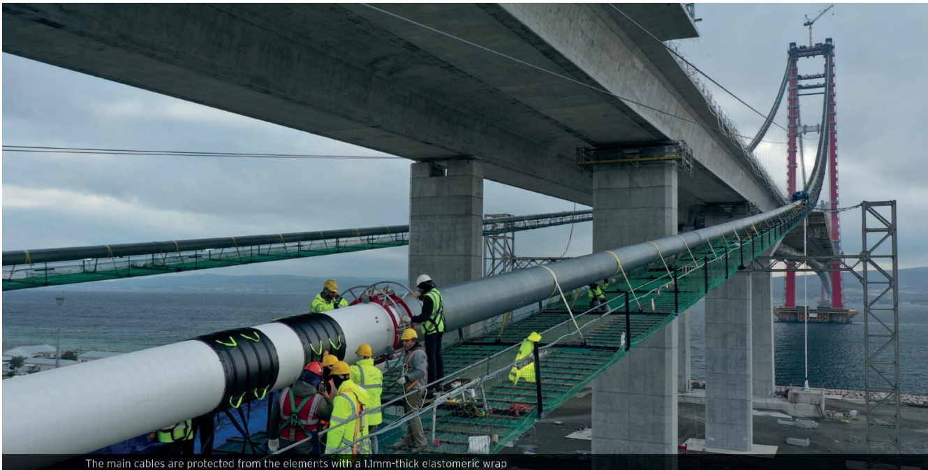
The main cables are protected from the elements with a 1.1mm-thick elastomeric wrap
