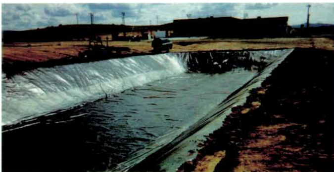
Oily wastewater holding pond, U.S. Forest Service, Prescott, AZ.
